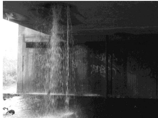
A leak from the flyover due to heavy rain.
