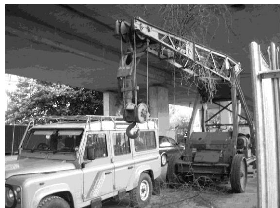
The crane as we received it. Peter Binns is removing branches from the jib.
